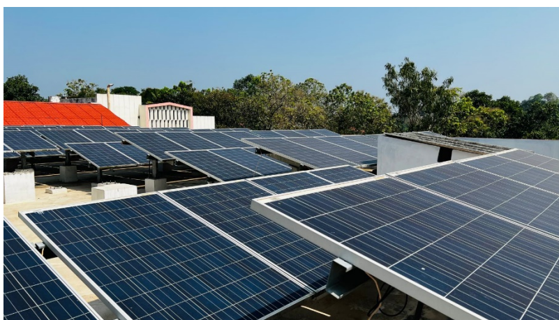
50kWp Solar power plant
