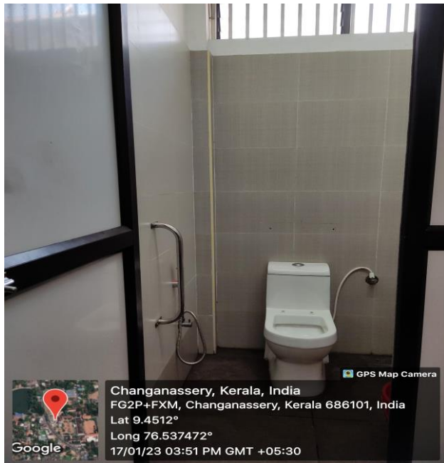
Geotagged photo of Divyangjan Friendly Wash rooms
