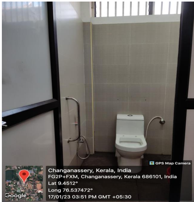
Geotagged photo of Divyangjan Friendly Wash rooms
